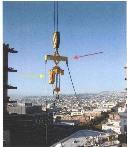
Red Arrow: Spreader Bar keeps rigging separated from electric chain hoist and handles 2/3 of the weight of the table, thus reducing the angle of the compensator and enabling the hoist to work more efficiently. Yellow Arrow: chain bag always faces the exit of the building. The back cables that go to the counterweight always keeps compensator facing correct direction. (Pictured right)
