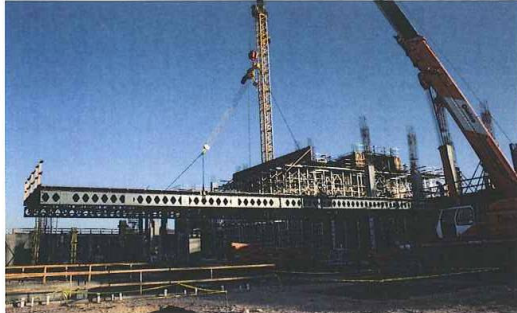
Pictured Left: Marnell Corrao, Project M in Las Vegas, Nevada. Signal-Rite Compensator is being used to pull 90 foot long, 31,000 pound tables. Project value is 700 million dollars.
